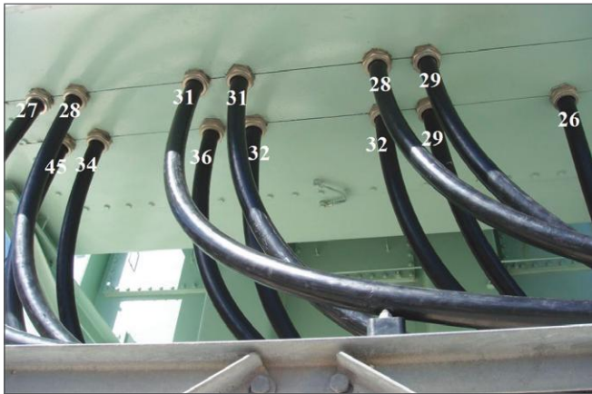
Figure 1 (the number superimposed on each cable represents the measured TEV value in dBmV)
