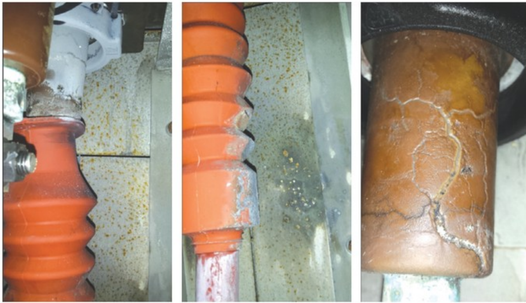
Switch No. 1 - Photos received from client April 2017
